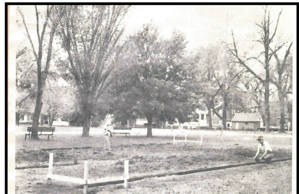
Ground has been broken for the new shelterhouse at Ellsworth. The 24' x 48' frame building will be located at the southwest corner of the park and will feature a 4' walkway all the way around, a 4' overhang, and a four way roof. Clarence Danger, on the left, and Steve Amundson are shown as they stake out the building.
